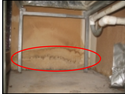
Stain on drywall in utility closet.
