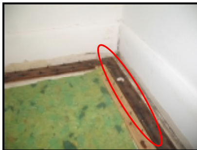
Water stained carpet strips in master bedroom closet.
