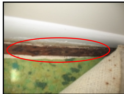
Water stained carpet strip at back porch exterior door.
