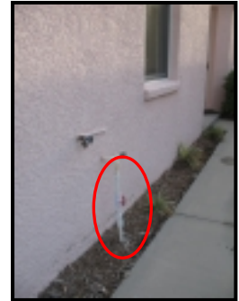
Main water supply valve
