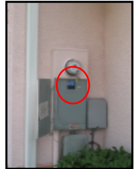
Electrical main disconnect
